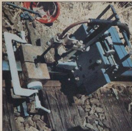
Fig. 2—Using a consumable guide and a self-shielded flux cored electrode, a mechanized vertical-up welding system joins the web and top flange of the rail.
