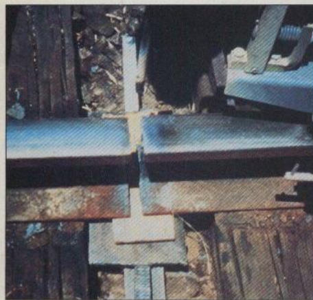
Fig. 3—To prepare a clean weld area, the rail joint is cut with the plasma arc process.
